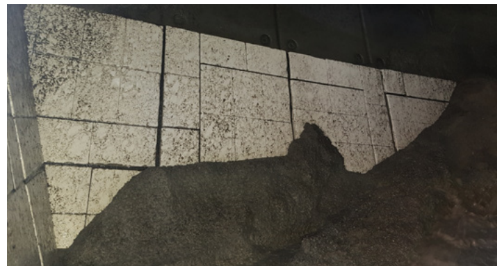
ProTech™ PT-92S ceramic liners in a rail carriage feed hopper.
